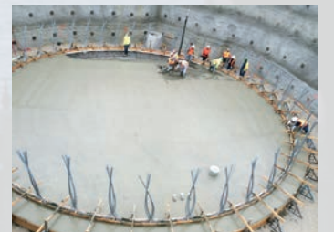
The Alta Vista Water Storage Tank, shown under construction here, was completed in 2016.
